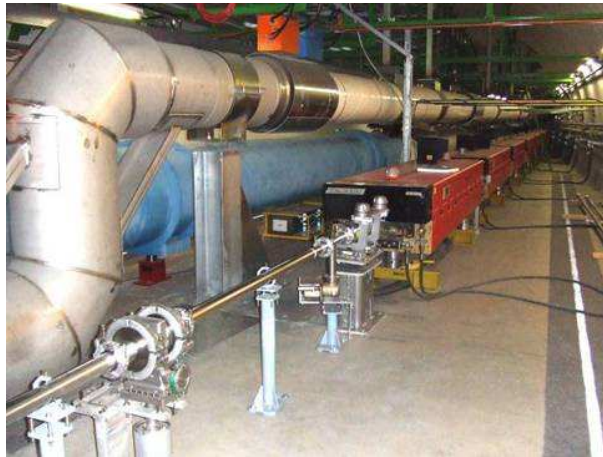
Figure 7: Junction of the injection line at Point 2.
