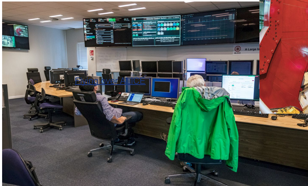
ALICE control room
